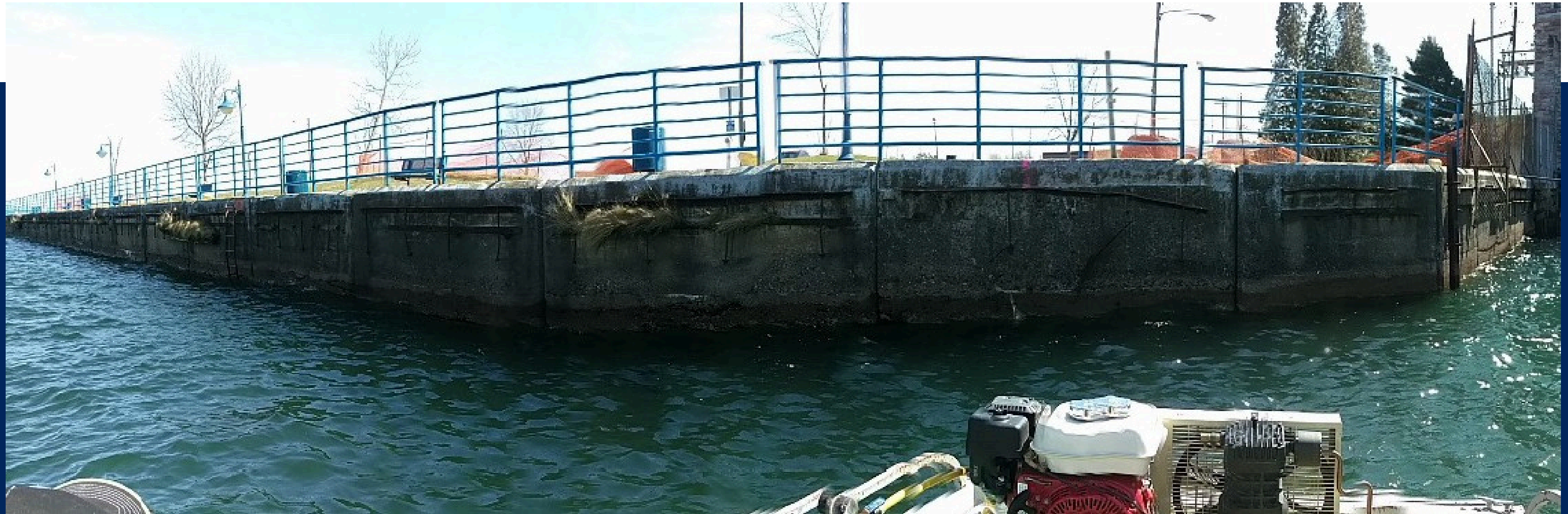
Deteriorated seawall and structural instability prior to rehabilitation
