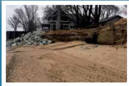
Riprap (large stones interlocked together to act as a barrier against erosion) in St. Joseph.
