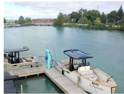
Elk Rapids Marina – Electric boats & charging infrastructure
