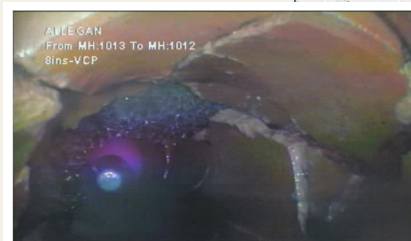
Figure 2. Multiple Fractures and Voids Identified in Sanitary Sewer Pipe in Project Scope.
